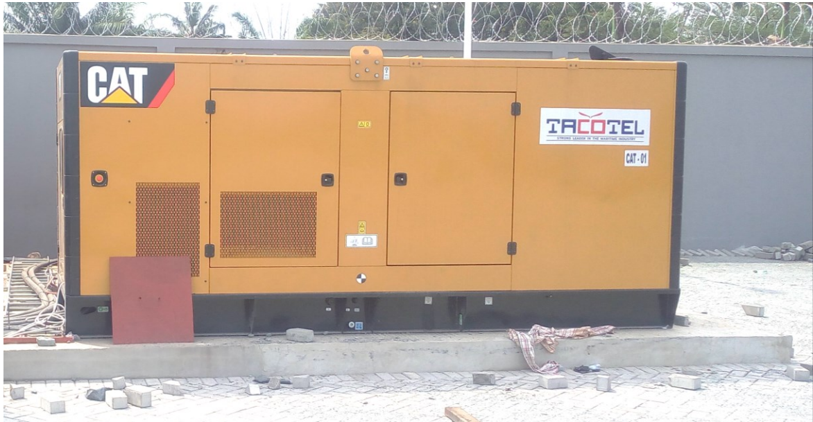
Figure 2-7: Outdoor generator with weather resistant coating
