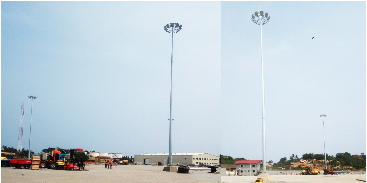
Figure 2-4: Some lighting fixtures in container area
